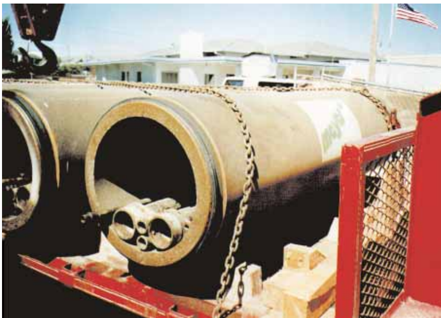
Delivery to site of the 24½ in diameter polycrystalline pipes from Meyer Germany.
