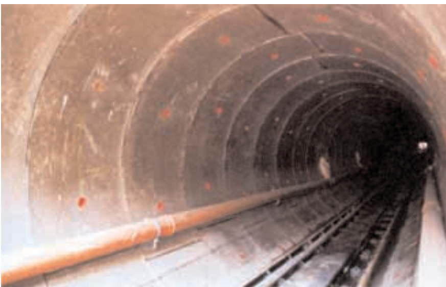
1 The world's first sewer made of polymer concrete tubbings is located in Offenbach / Main. (photo: tis)
