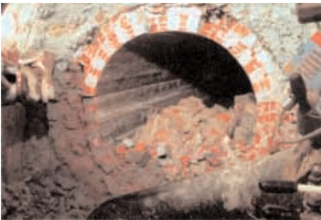
2 During the driving phase the house connections are cut and transferred to a temporary auxiliary line (photo: Meyer Rohr+Schacht)
